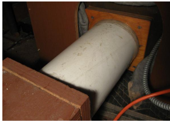
Figure 31: PVC pipe used to connect the blower to the plenum.
