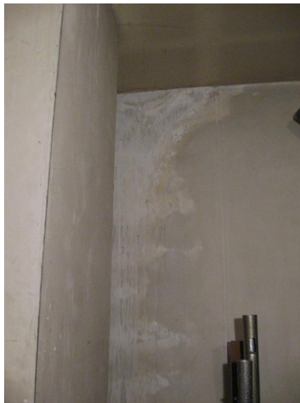
Figure 21: Swell division, left front, showing flaking plaster
