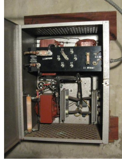
Figure 48: Inside the rectifier, showing it is set for 15 volts DC.
