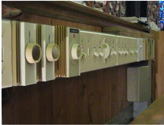
Figure 15: An extremely large number of lighting switches and rheostats, clearly intended for the organist to control.
