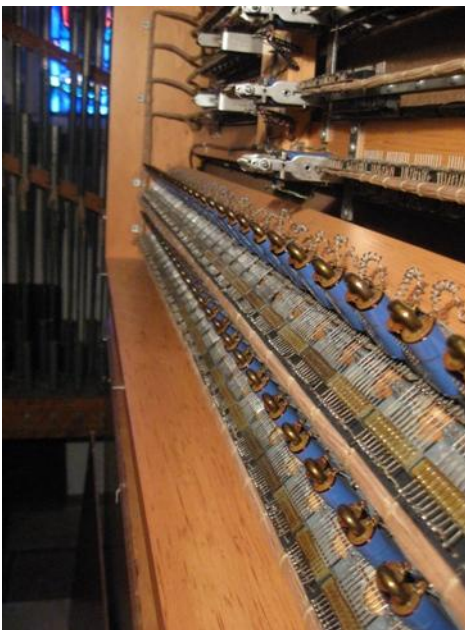
Figure 46: The relay, also called a Switching System.
