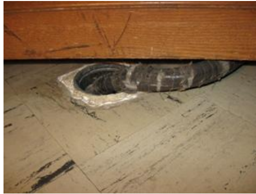
Figure 14: The cable, or umbilical cord, connecting the console with the relay. Note its tenuous condition.
