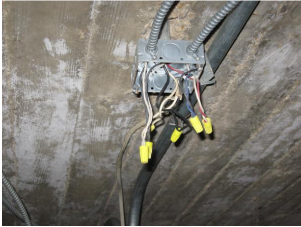
Figure 49: open electrical box.
