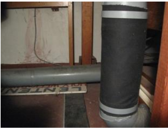
Figure 30: Painted, galvanized steel windlines (grey) and rubberized cloth sleeve (black).
