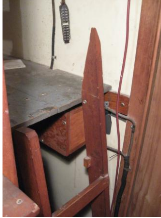
Figure 54: dangerous ladder in Great chamber.
