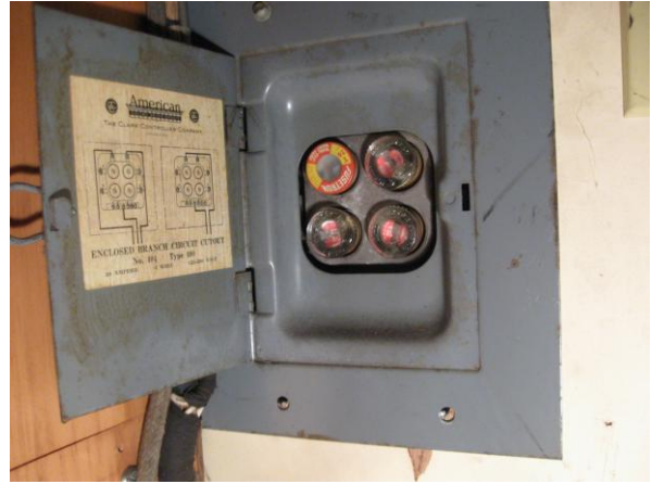
Figure 50: Electrical box with screw-in fuses.
