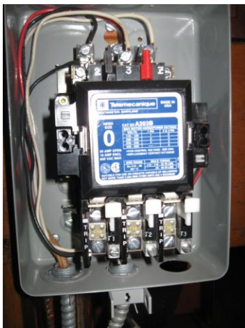
Figure 16: The contactor for the blower motor
