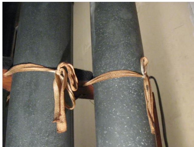
Figure 39: Large zinc pipes held in place with cotton twill tape.
